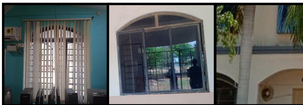
Ventilation and Exhaust system Facilities in MAMSE Buildings
