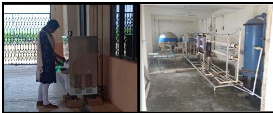
Water supply units and treatment facilities at MAMSE, Tiruchirappalli, TN
