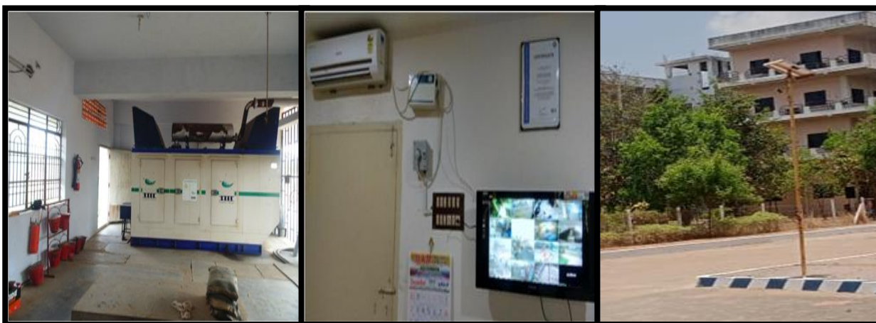
Energy Conservation and Management Activities at MAMSE, Tiruchirappalli, Tamilnadu.
